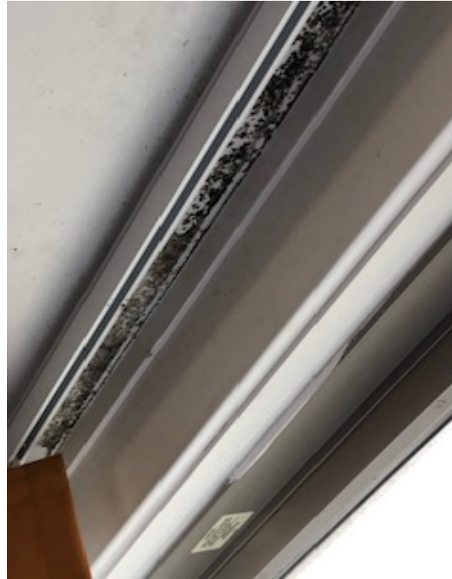
Mold On Curtain Track
