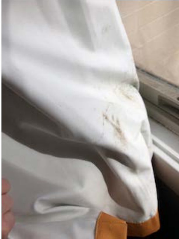
Mold on Inside of Curtain
