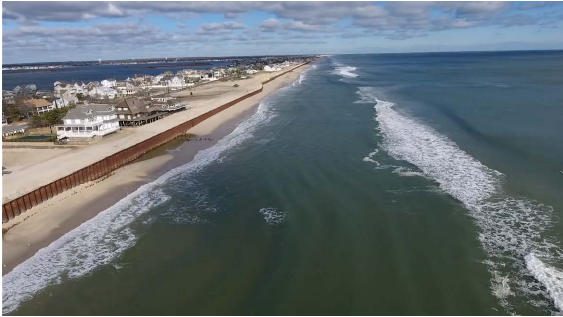
Aerial view looking north along Mantoloking following a moderate northeast coastal storm in January 2017. This storm caused extensive beach erosion exposing the steel wall installed following Sandy. (Aerial photo courtesy of Ms. Jenny Buck)
