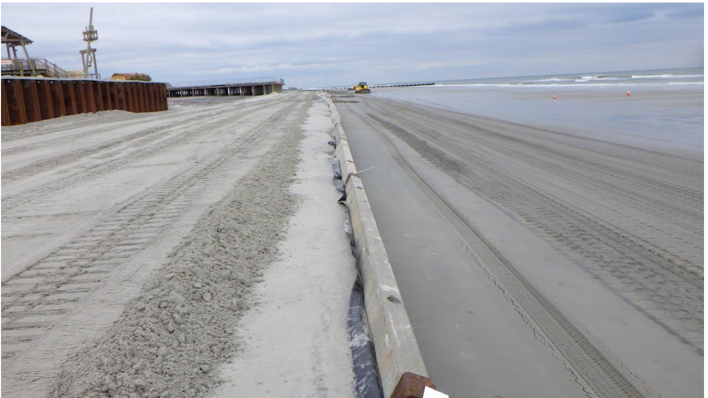
Figure 24. View to the north taken on January 27, 2021 looking along the concrete “Jersey barriers” employed to retain the sand for the road. Seaward the beach is extremely flat, but quite wide. Waves easily reach the bulkhead making a dry berm unlikely until the shoreline advances seaward about 100 feet further seaward.
