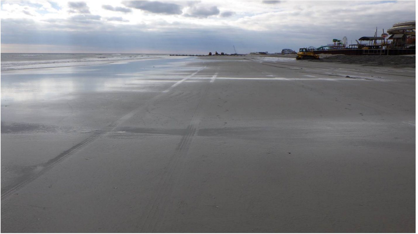
Figure 22. Site 60+00 lies between Morey’s Surfside Pier and the next timber pier to the north. The bulldozer is maintaining the haul road entrance past the two timber piers.
